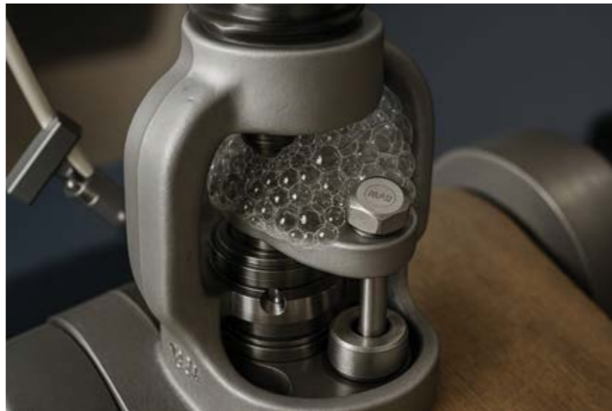
Leaking stem seal during a fugitive emissions test.
