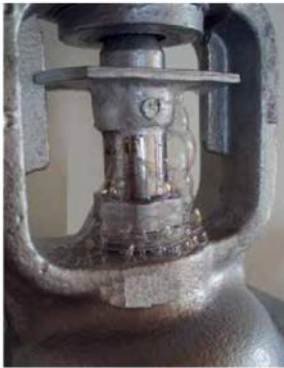
Stem leakage due to leaking bellow during valve pre-testing
