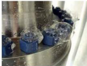
Leakage of body gasket via bolting
